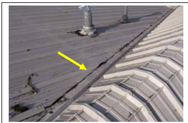
North Valley Leaking
