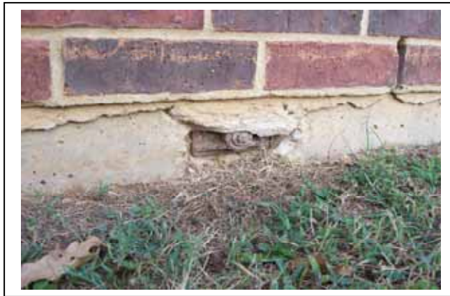
Exposed tension cable needs to be sealed.
