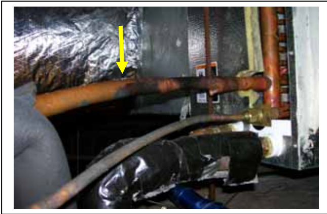
Insulation on the refrigeration lines needs to be replaced.
