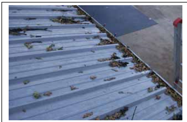
Gutters need to be cleaned.
