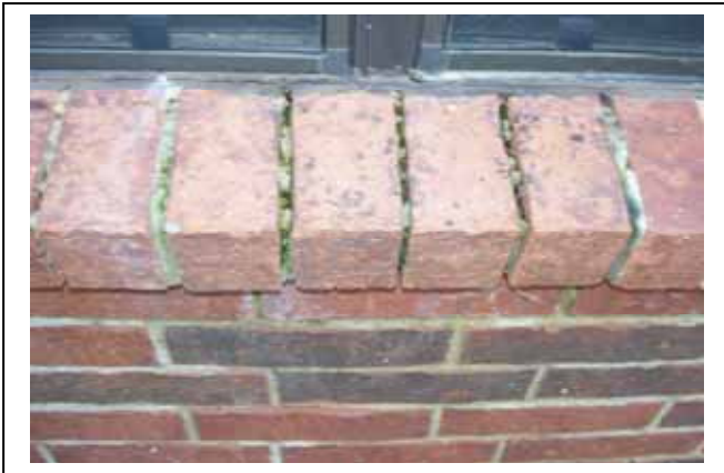
Window seat mortar needs to be improved on the north side of the structure.
