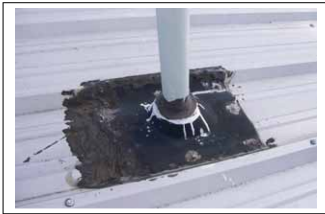
Improper roof jack installation.
