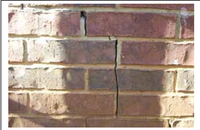
Mortar improvements are needed on the south side of the structure.
