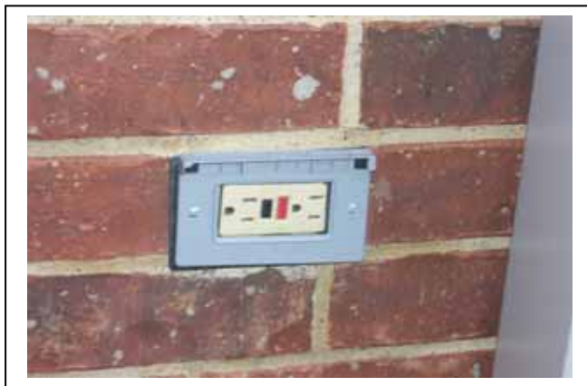
Receptacle weather cover is missing.
