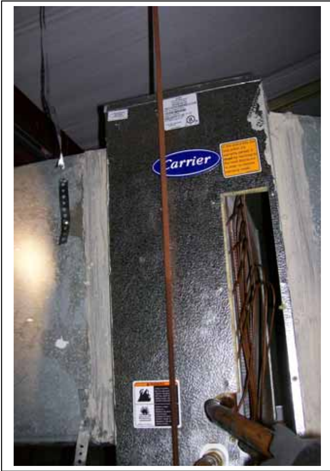
Coil service panel is missing to unit #2
