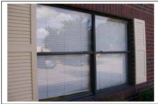
Window screens are missing.
