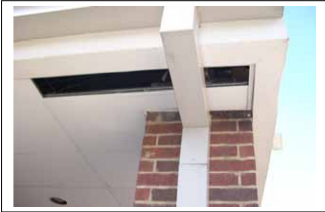
Carport soffit panel is missing.
