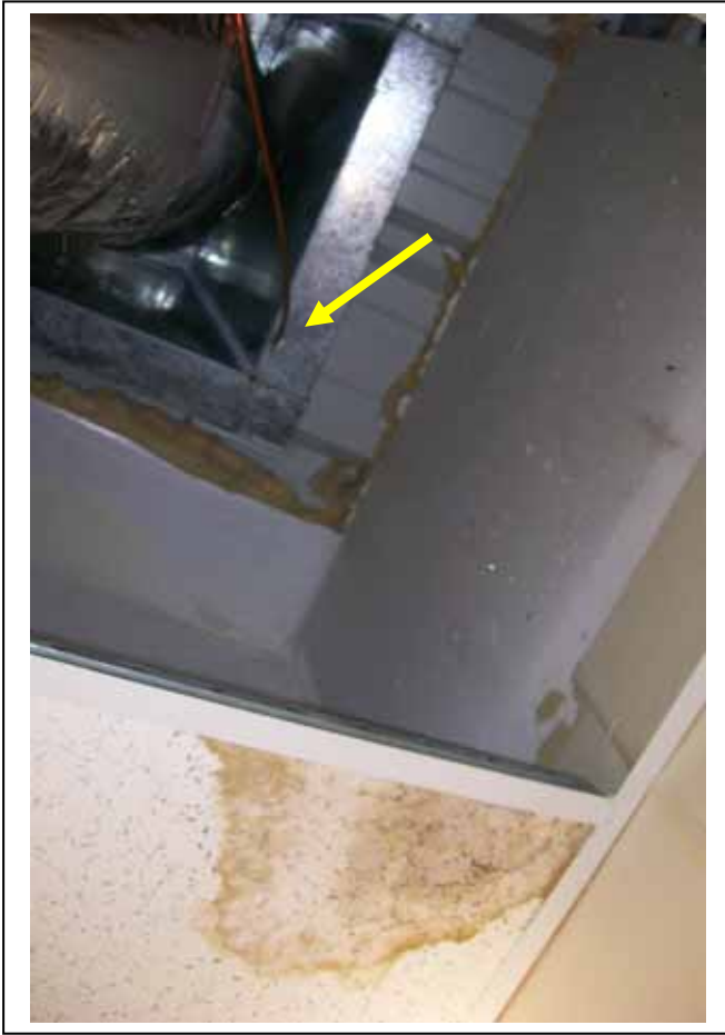
Roof leak over the southwest classroom restroom area.
