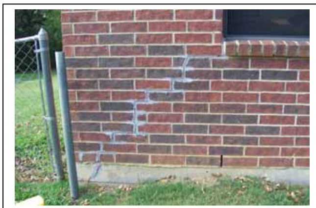
Prior mortar repairs on the north and south sides of the structure.
