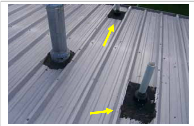
Improper roof jack installation and prior repairs
