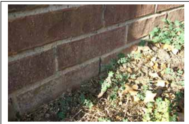
High soil line on the south exterior wall.
