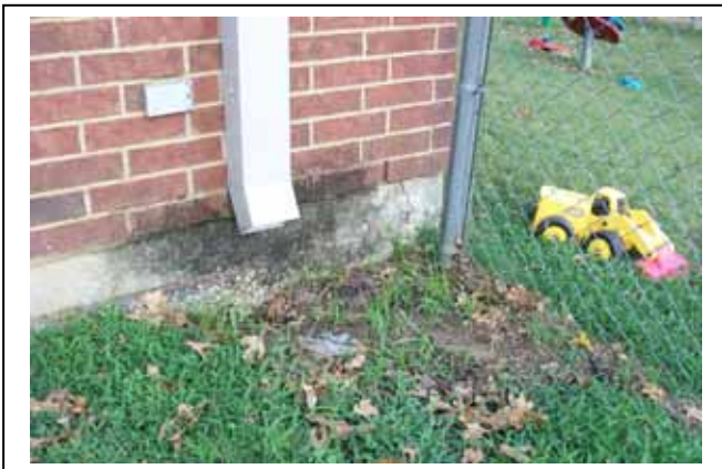
Downspout splash block is missing
