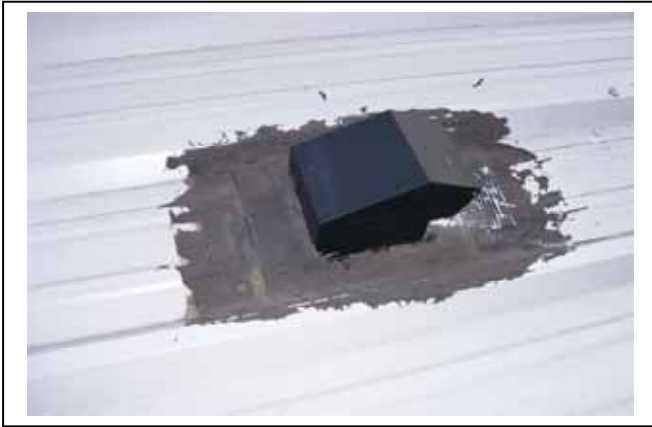
Improper roof jack installation.
